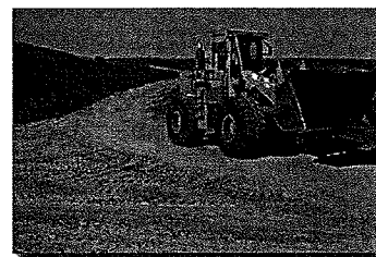
Figure 13. Road dust after applying polymer flocculant
